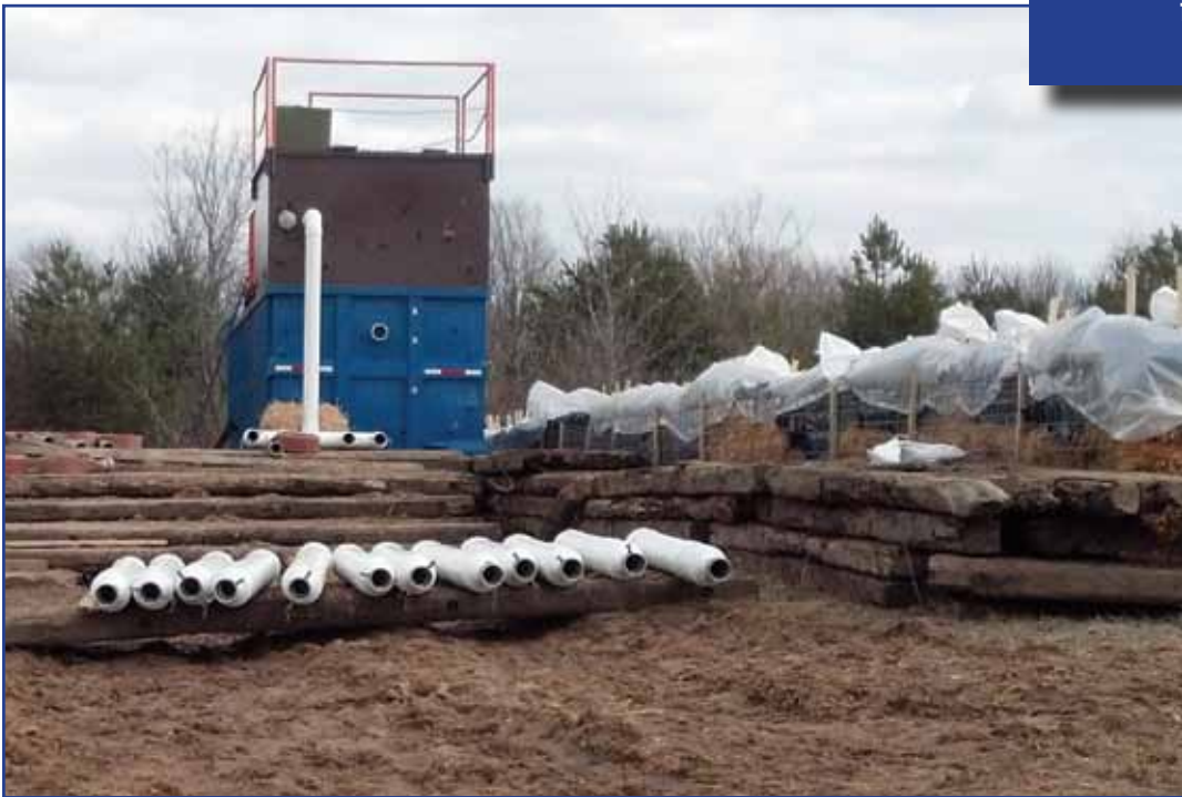
Water Matrix setup next to pond #1 with first bank of Floc Hogs.
